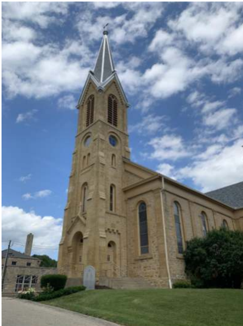
St. Norbert's Catholic Church, Roxbury, WI exterior restoration assessments, estimates, design documentation and repair oversight of stabilizing the church bell tower, Replacing the slate roof, substantial masonry repairs & window restoration.
